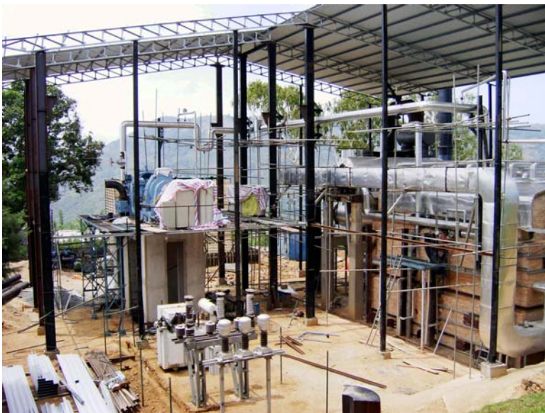
1 MWe Biomass-Fired Boiler-Steam Turbine System feeding the National Grid
